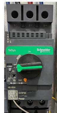
Heater Overload Tripped (OFF)
