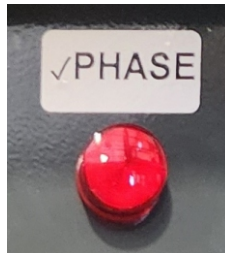
PHASE ALARM LIGHT - ON
