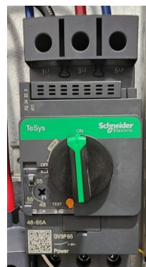
Heater Overload ON (Reset)
