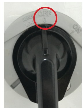
7. Main Power Switch in OFF Position
