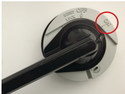
2. MAIN POWER SWITCH in ON Position
