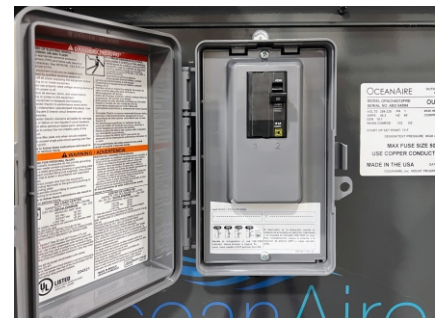
MAIN POWER BREAKER (COVER OPENED)
